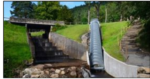
National Trust's Archimedes screw micro-hydropower at Cragside, Northumbria
