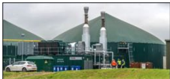
Agrivert food-waste digesters and 2.4MW generators, Crowmarsh, Oxon
